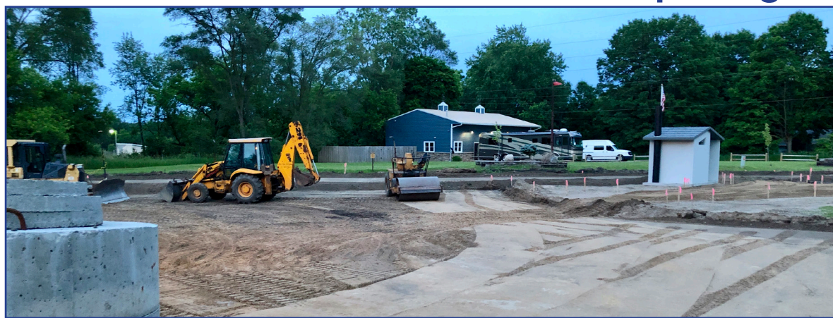
Parking lot complete with restroom constructed next to M-52/M-106 on the south side of Stockbridge. Photo credit Patrice Johnson
