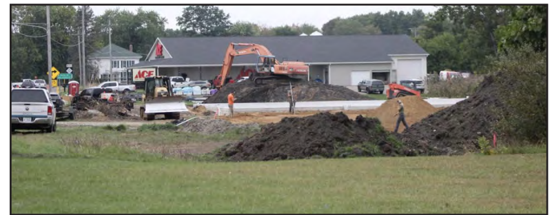
The Tractor Supply Co. is expected to be finished by the summer of 2024, and the Dollar General Market is expected to be finished by the end of 2023. Photo credit Evan Sandecki
