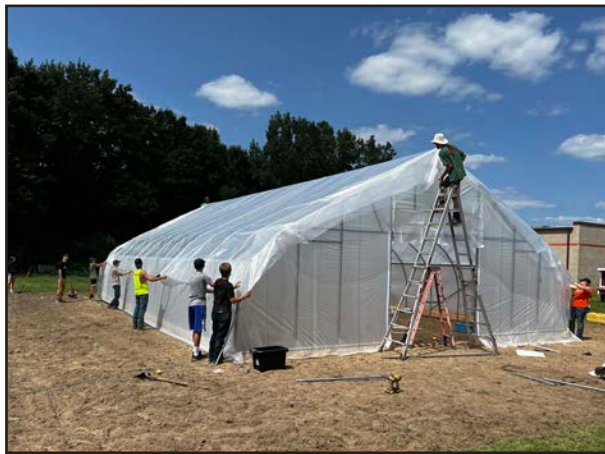
The top of the hoop house frame is covered in plastic. Photo provided by teacher Bob Richards
